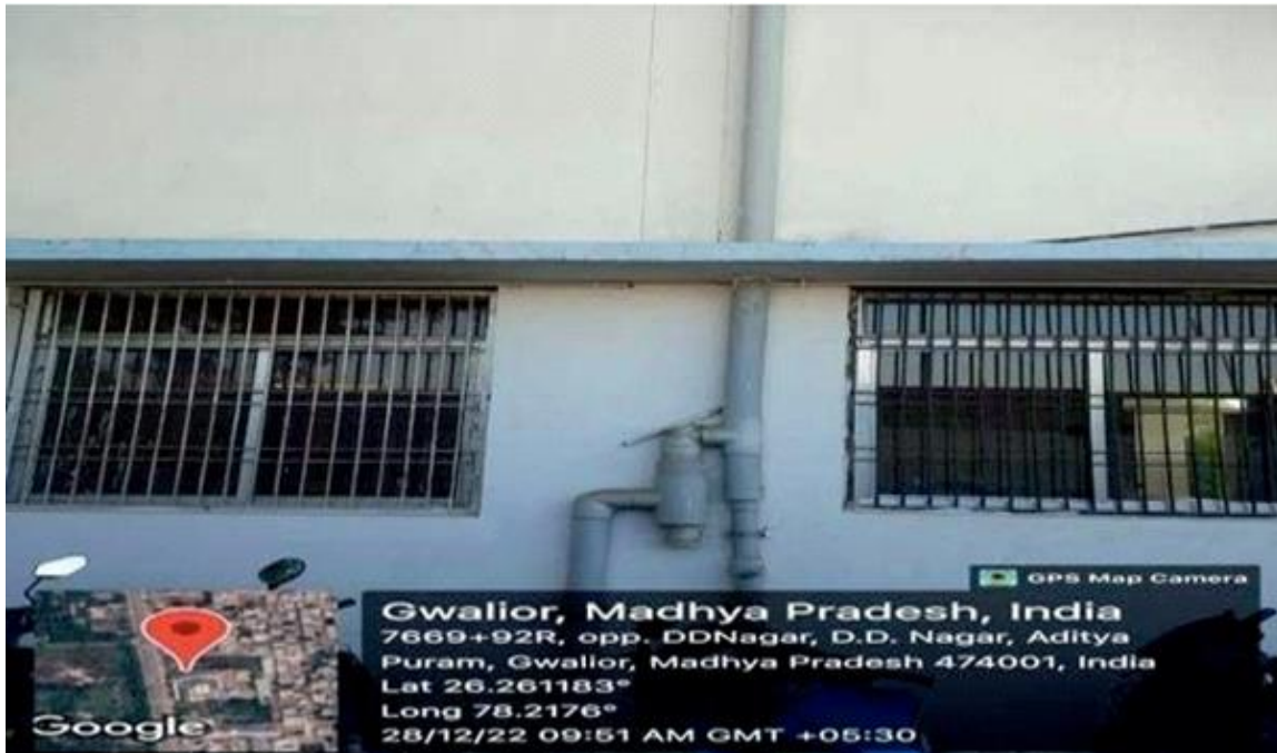
Rain water harvesting pipe System Block B
