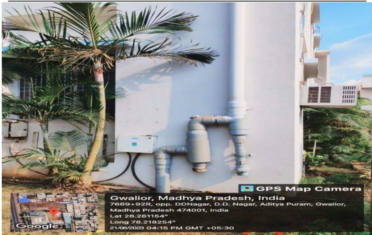
Rain water harvesting Pipe System at Block A
