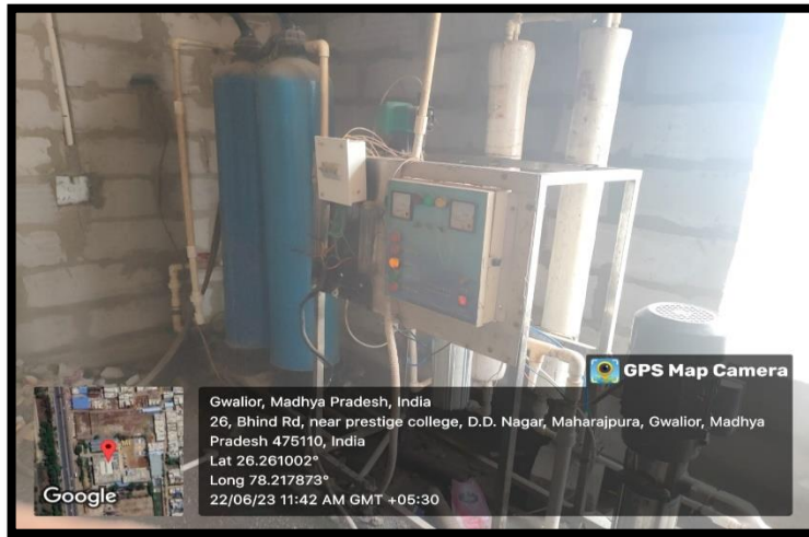
RO Waste Water collection in the Tank for Reuse
