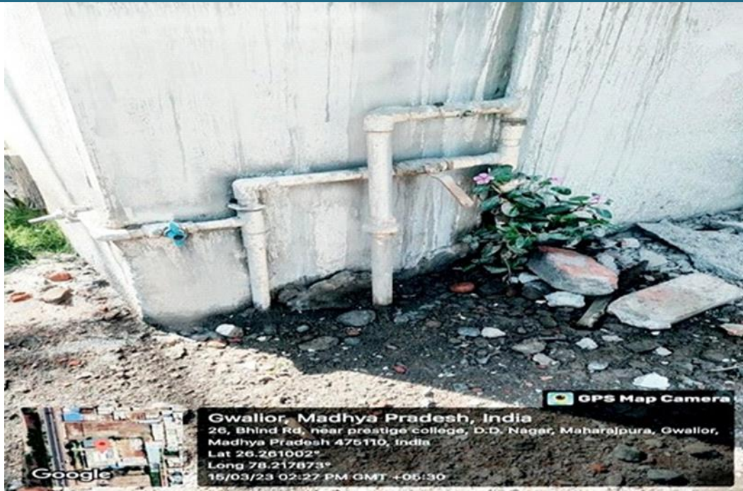
Water Distribution Pipe System in Block A
