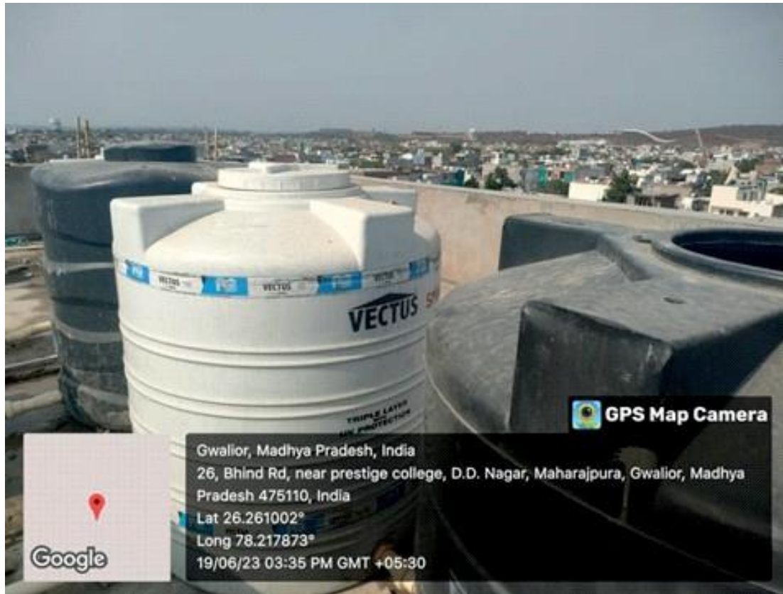
Water tanks at Rooftop of Block C
